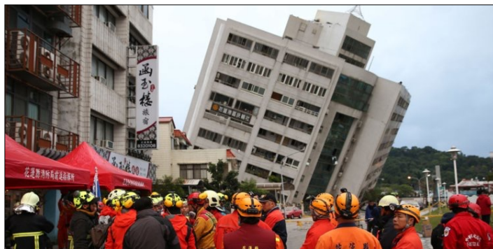
A building tilts to one side after a 6.5-magnitude earthquake on Feb 7, 2018 in Hualien County, Taiwan. Unioncom/VCG via Getty Images
